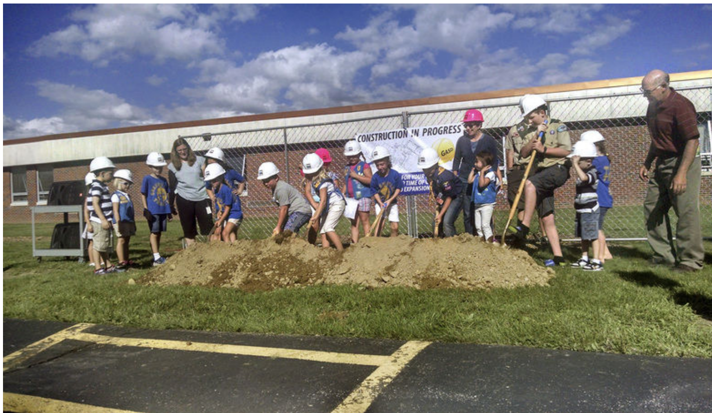
Greenville school board President Dennis Weber, right, oversees youngsters breaking ground for an expansion of Hempfield Elementary School. LYNN SATERNOW | Herald
